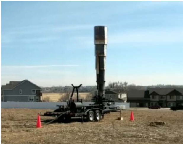
VOC Emission Control Unit
